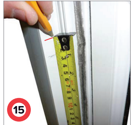
15 Carefully measure 20mm up from the pencil line and mark the outer frame.
